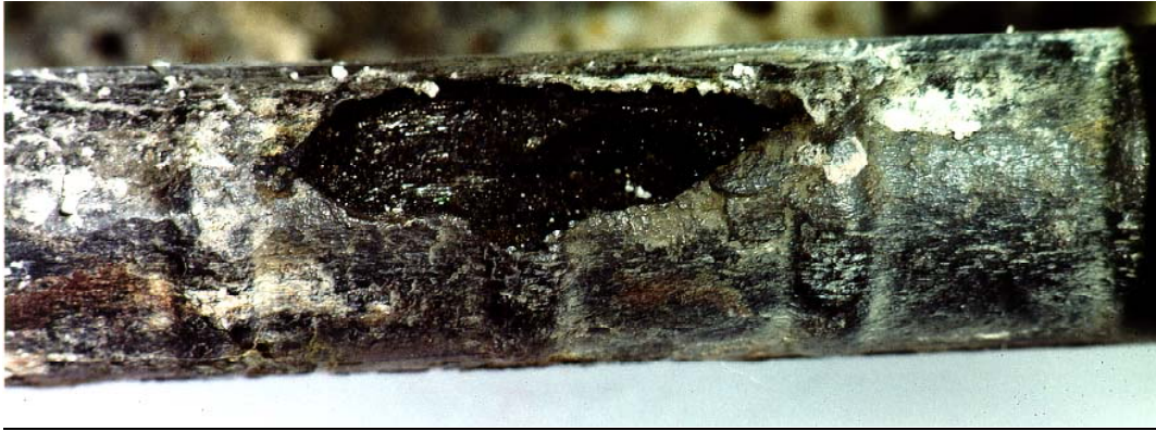
Figure 1 : Localized corrosion attack on a 20 mm rebar, loss in cross section ca. 30%
